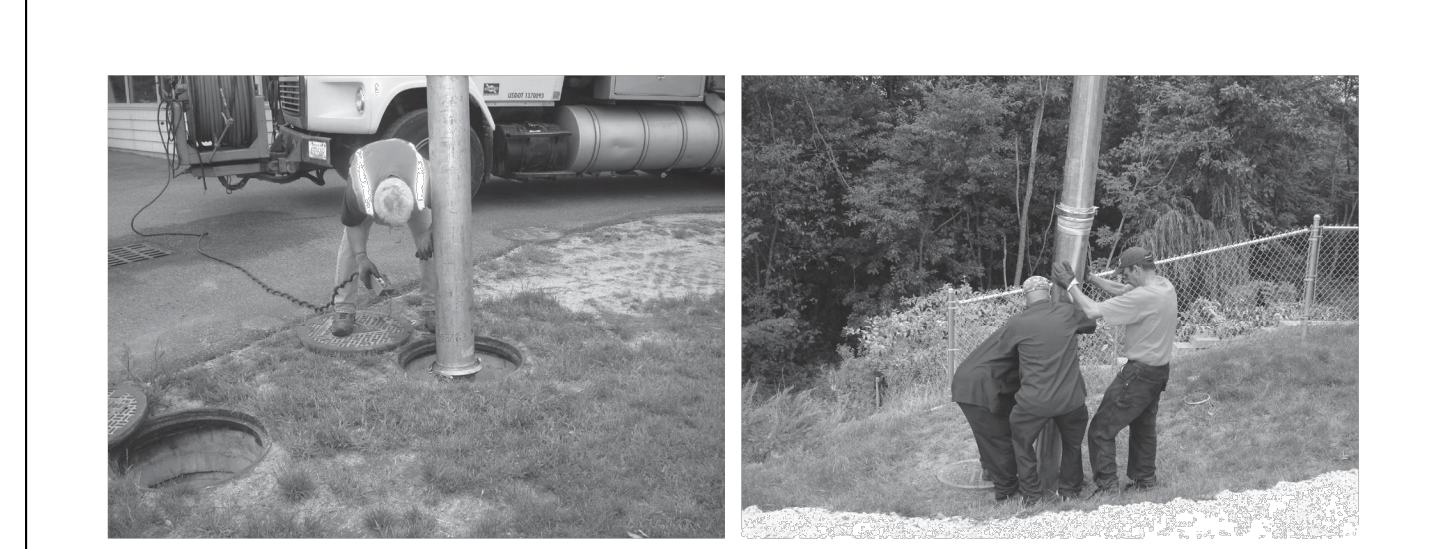
A Cascade Separator unit can be easily cleaned in less than 30 minutes. A vacuum truck excavates pollutants from the systems.
