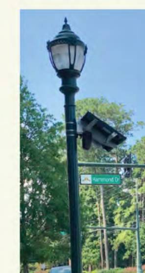
Solar & Existing Pole
