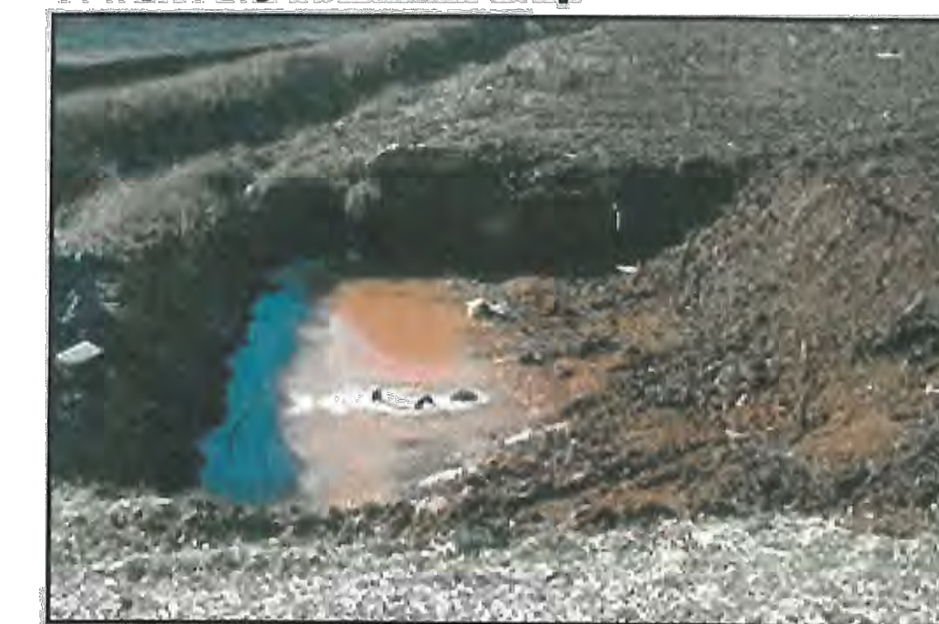
Figure 6.73 Sediment traps are used to collect sediment laden runoff from disturbed areas on construction sites. (Source: EPA)
