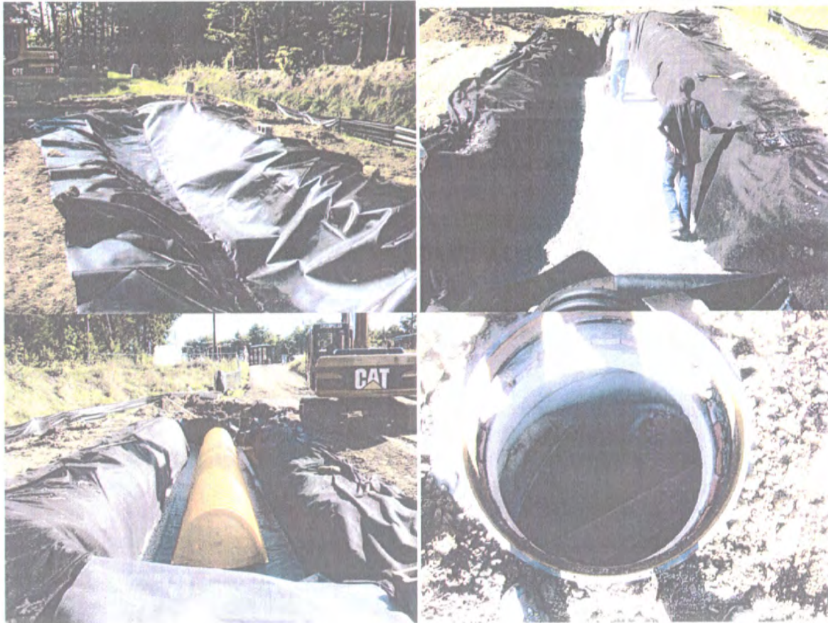
Figure 2: Installation of Isolator Row September 2006; (a, top left) HDPE liner installation to monitor full treated effluent; (b, top right) Crushed stone subbase 12" thick installation; (c, bottom left) Installation of Isolator Row chambers on top of double layer of woven geotextile fabric (bottom) non-woven geotextile fabric (sides) and stone subbase; (d, bottom right) Installation of hydraulic inlet structure, chamber entrance (left), influent source (top right), and high flow bypass weir bottom right.
